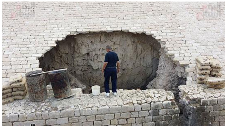
Fig (4): The hole on the northern wall of the citadel. Source: Based on photos of El-Youm El-Sabea Journal (accessed on 23, Sept 2020).
